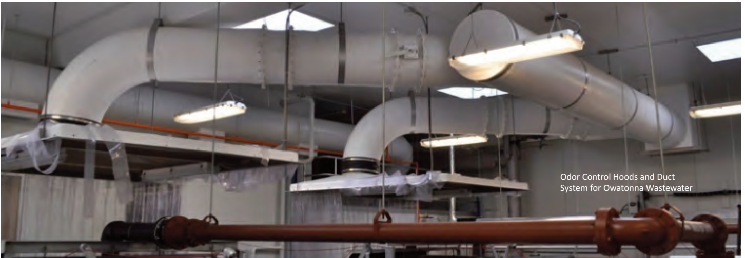
Corrosion Duct System
